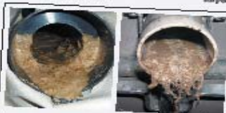
Struvite is the main scale material that builds up immediately downstream of waterless urinals, causing major blockages when not properly managed. These pictures show the build up of struvite within 12 months of installation.
