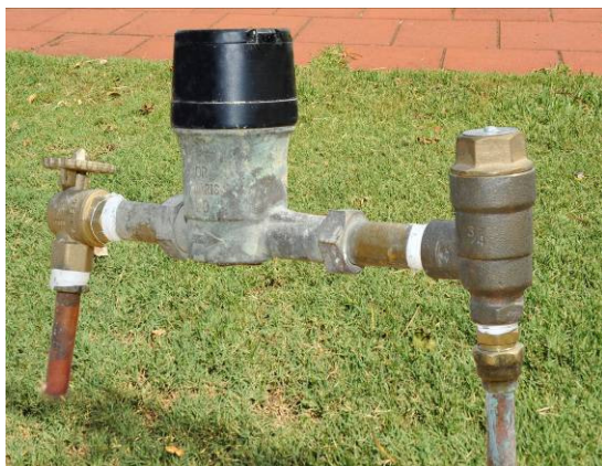
Pressure Reducing Valve installation
